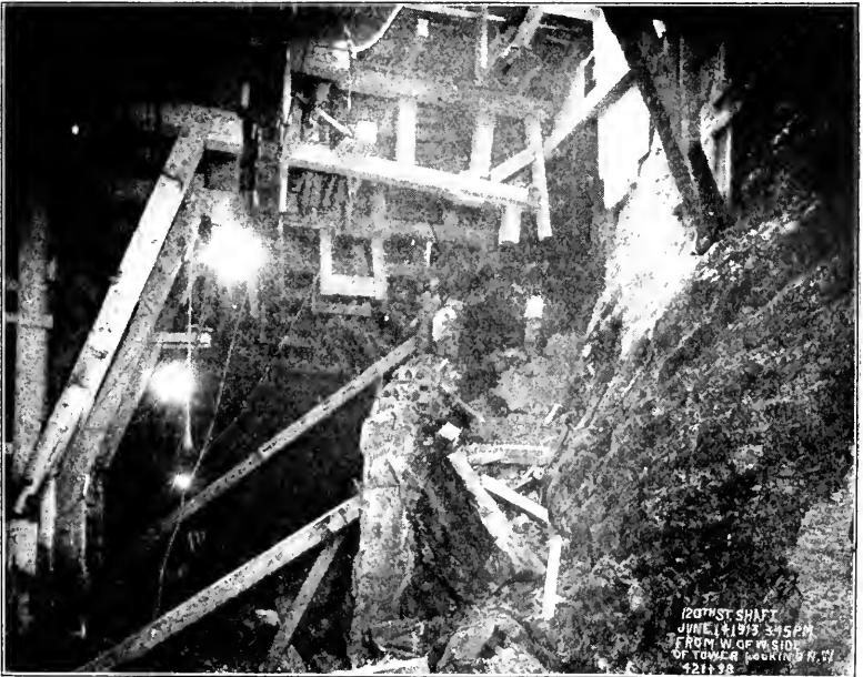
FIG. 2.—TYPICAL ROCK SLIDE, IN LEXINGTON AVENUE.
